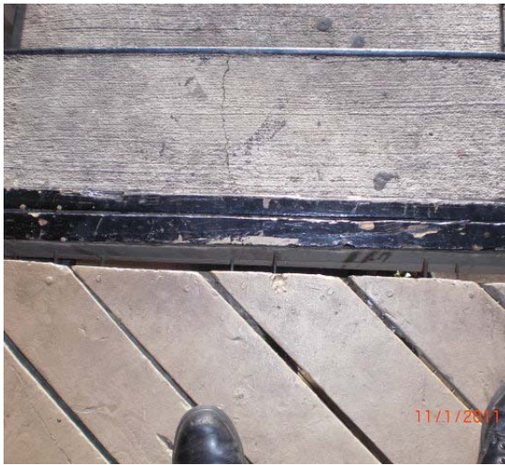
Stairway being held up only by nails and pulling away from walkway.
