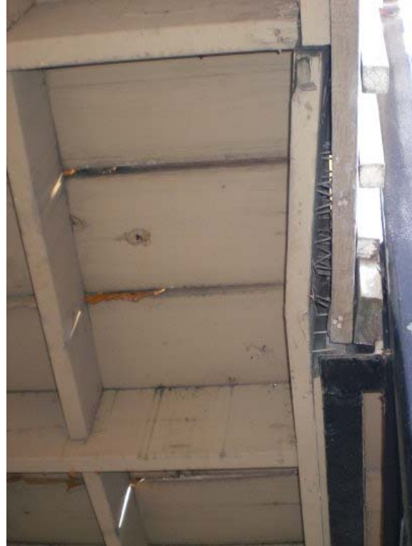
Second floor walkway becoming detached from support posts and at risk of collapsing.
