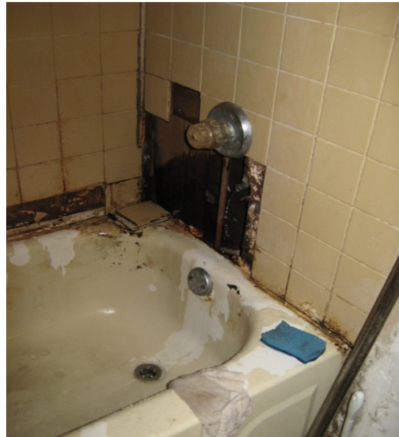
Missing tiles, rotting wall, mildew, and mold.
